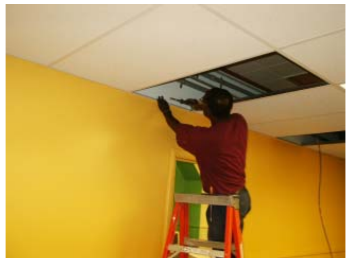
Henry electrician Nathan Awuah-Korang cuts a hole to run wire for new electrical outlets at Anchor Learning Center as part of this year's United Way Day of Caring.
